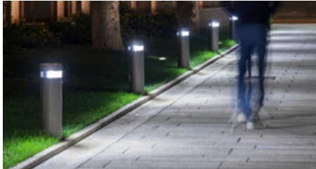
Bollard lighting along new paths and routes through the park
