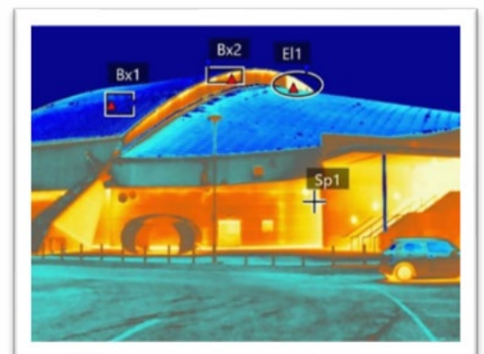
Figure 6, thermal photograph of the Velodrome showing heat escaping from the roof
