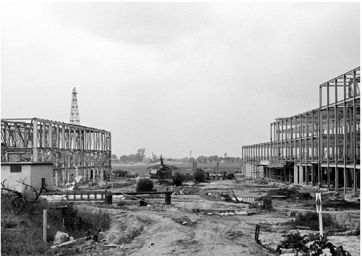
Photograph showing airport terminal during construction in 1961 - Source: Manchester Local Image Collection
